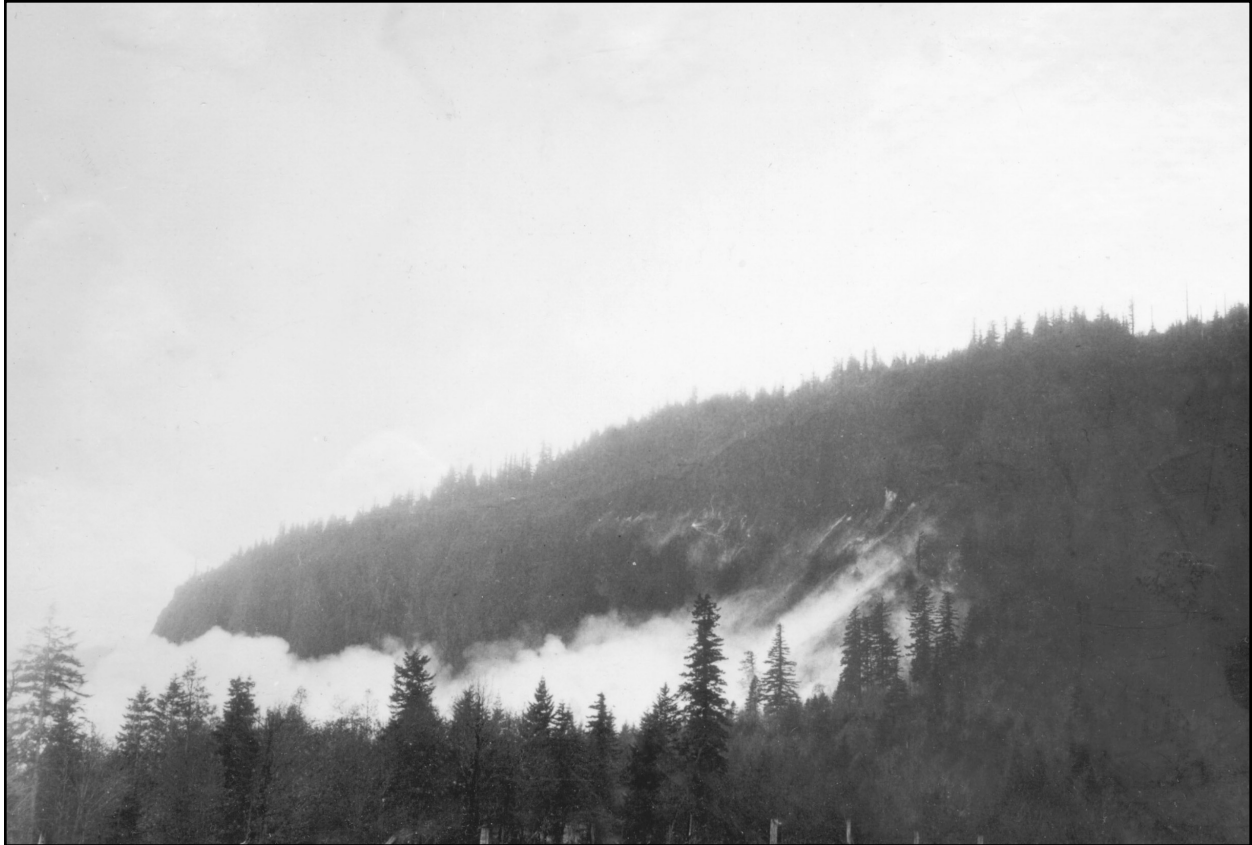
Puff of smoke goes up when the dynamite went off and the rock came tumbling down at Cape Horn.
